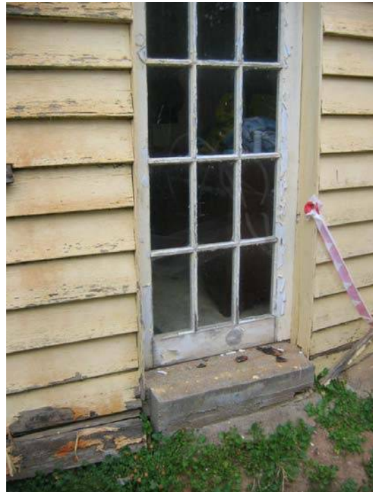
Poor amenity at door threshold
