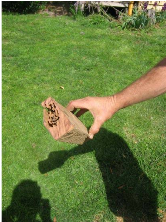
Evidence of termite damage to studs
